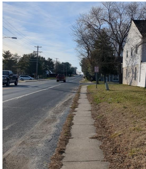
Figure 2: a picture showing the condition of some sidewalks on South Little Creek Road.
